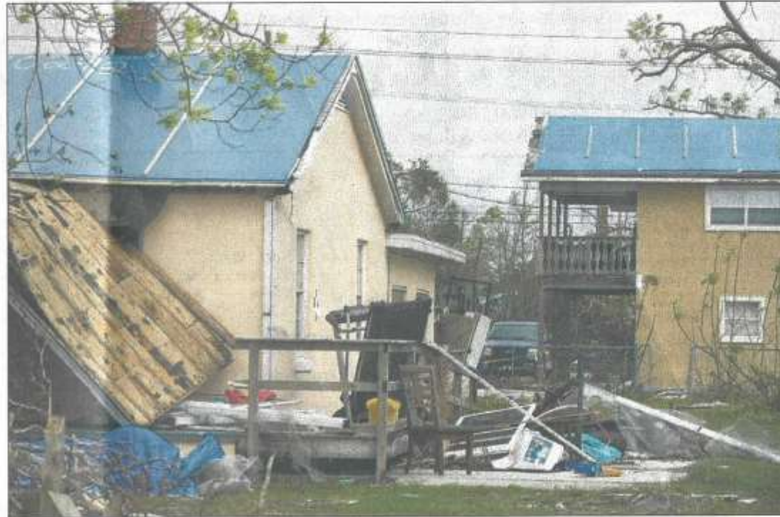
Homes damaged by Hurricane Michael, with blue temporary roofs, are seen on Nov. 15. [JOSHUA BOUCHER/ THE NEWS HERALD]
